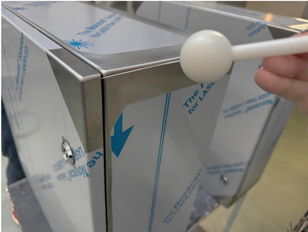
Photo 8 Enclosure protection, IP6X. 1 mm probe – Adequate clearance kept.
