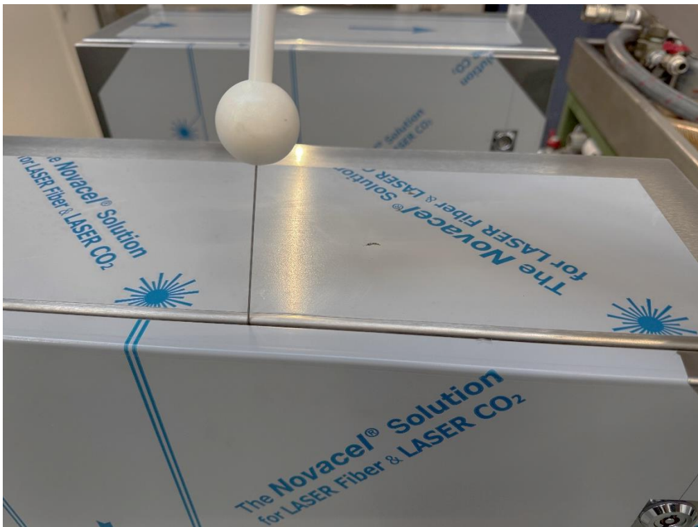
Photo 9 Enclosure protection, IP6X. 1 mm probe – Adequate clearance kept.
