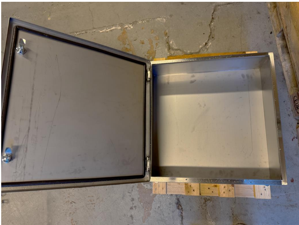
Photo 15 Visual inspection, IPX6. No ingress of water observed.
